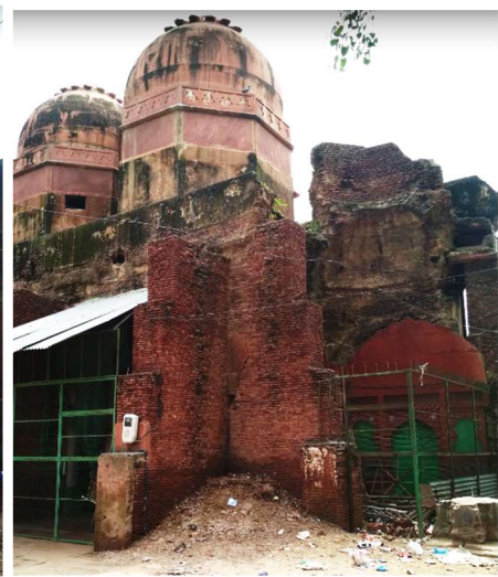
The image showing collapsed third dome of the mosque and temporary supports of brick masonry.
