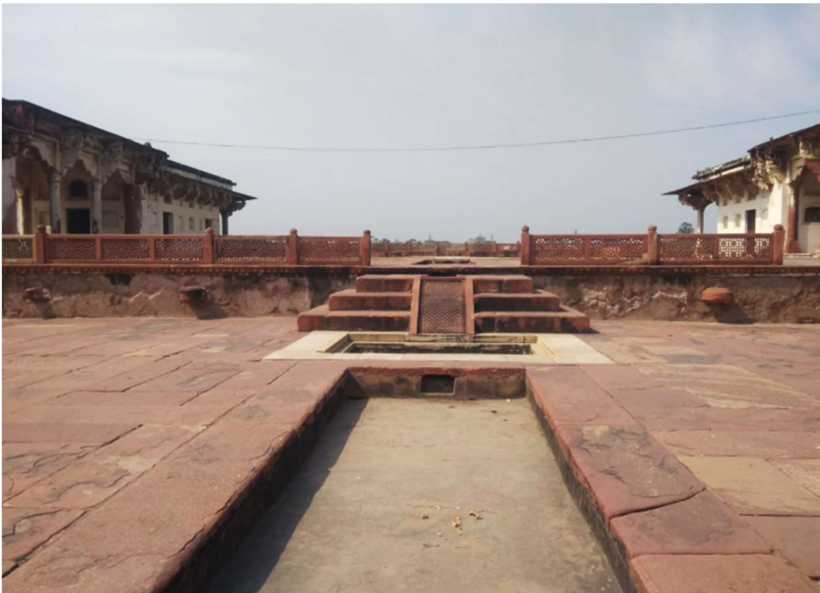
Condition of terraces of charbagh are stable. Signal storey houses are also in stable condition. There are signs of stone deterioration.
