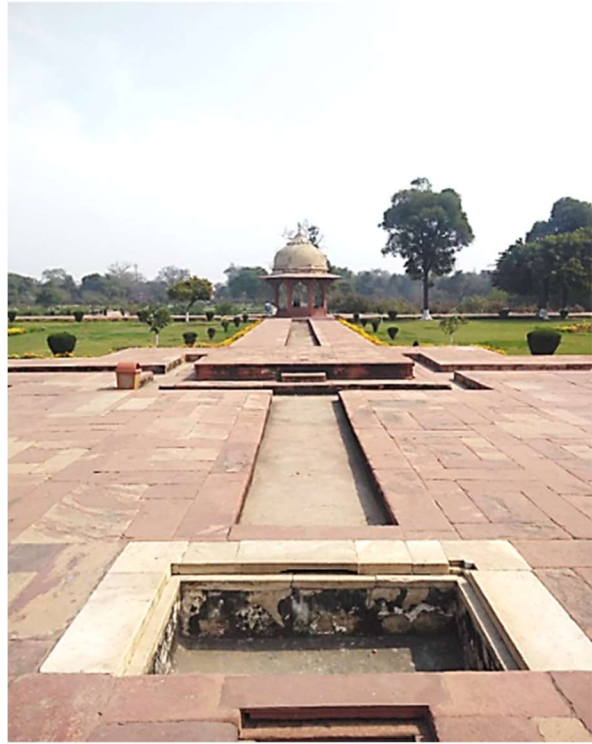
Condition of terraces are stable. There are signs of stone deterioration in patches all over.
