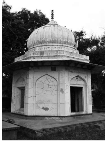
Plaster cracks on exterior surface
