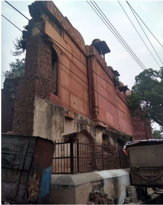
The view of mosque from north west direction showing a brick masonry supporting the mosque from further collapse
