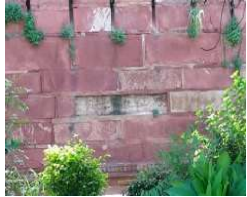
Figure 23: Loss of Cladding
