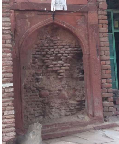
The loose masonry and deteriorated stones of the exterior wall surface
