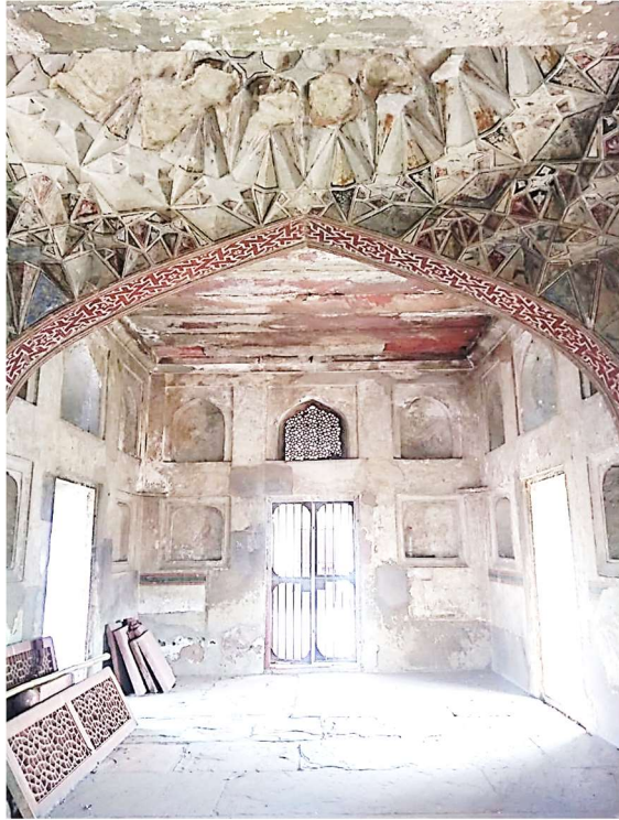
Decorative features in the interiors of pavilions showing sign of deterioration
