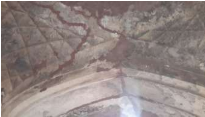
Figure 27 Cracks in the ceiling
