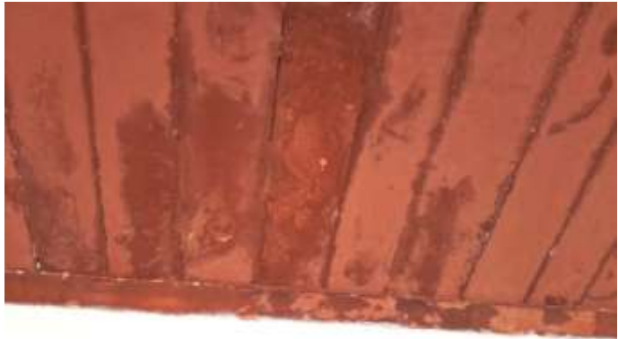
Figure 62: Water Ingress in roof
