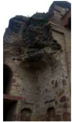
Figure 28: Vegetation Growth and structural damage
